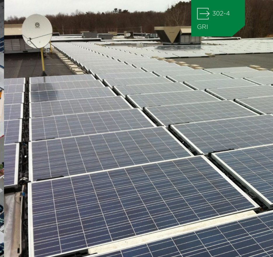
Shops at Saugus | Boston, MA | Regency Solar Array
