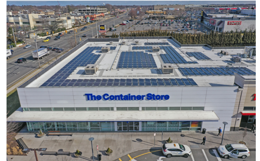
The Gallery At Westbury Plaza | New York, NY | Rooftop Solar Panels
