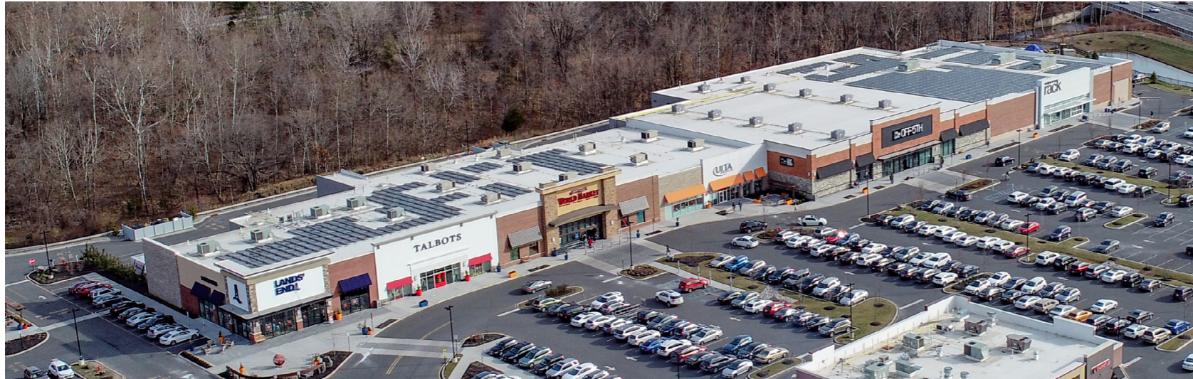
Chimney Rock | Bridgewater, NJ | Rooftop Solar Panels
